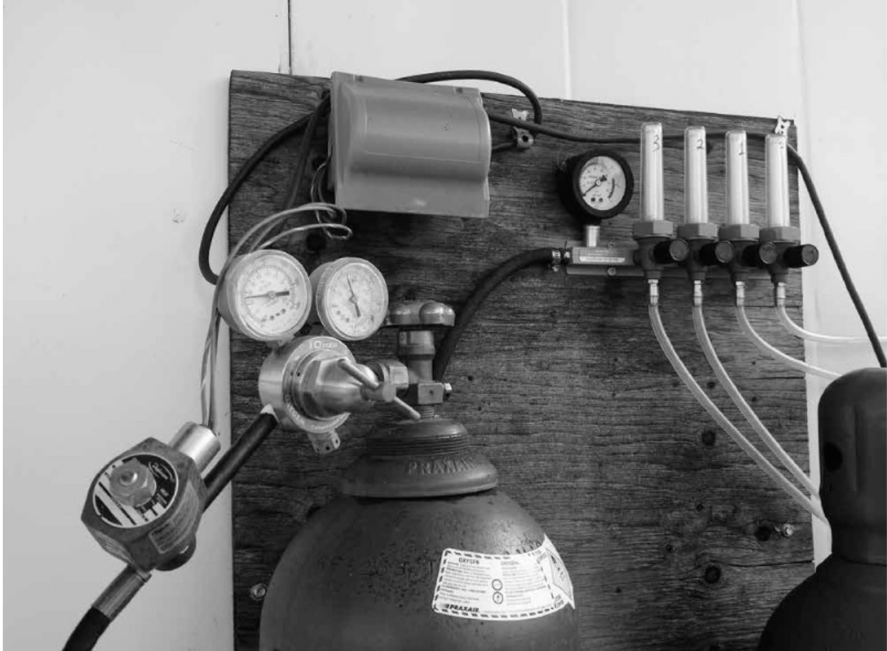
Backup oxygen system: oxygen tank, pressure regulator, solenoid valve and flow meter manifold.
