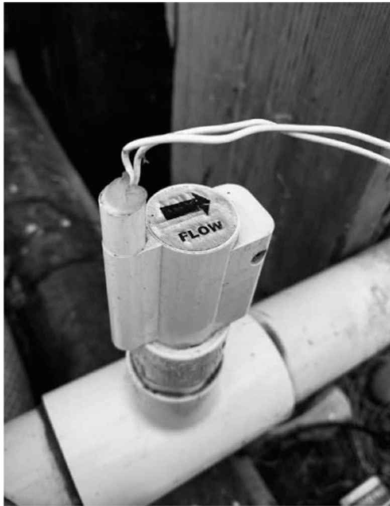
Aqualarm 10235 Flow switch.
