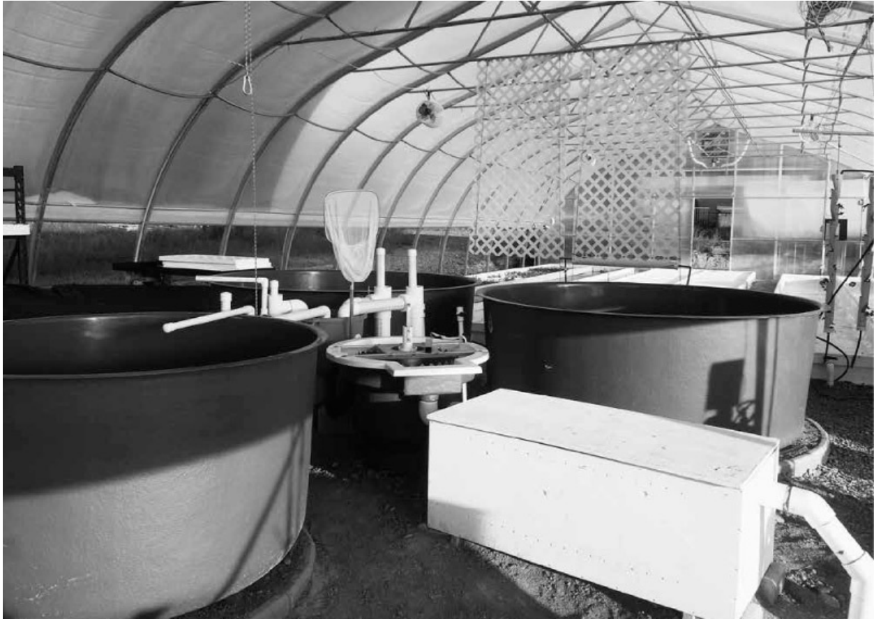
The fish tanks, Tank Manifold and filtration systems (RFS and CFB) at our farm.
