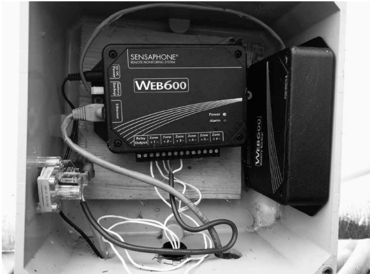
Web600 monitoring system with battery backup (right) and aeration pressure switch (left).
